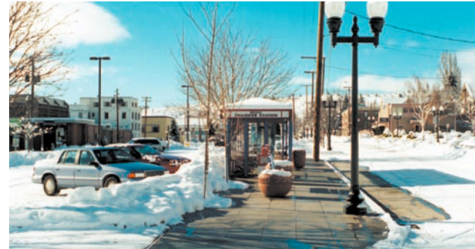
Klamath Falls, Oregon, a geothermal district-heating system keeps the sidewalks clear and dry at the Basin Transit station after a snowfall
