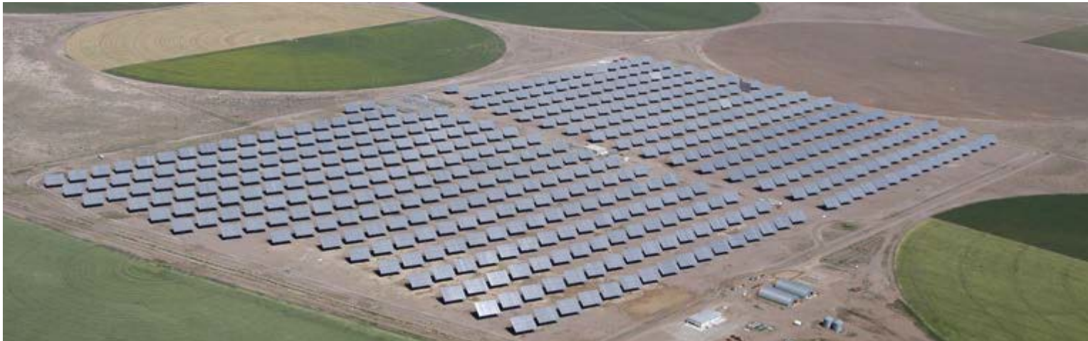
30 MW plant in Alamosa, Colorado, USA (© Amonix)
